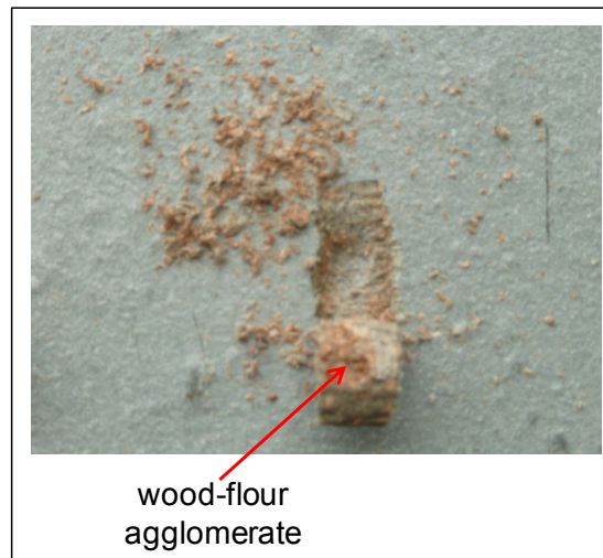
Figure 2.28 Photograph of wood flour scooped out of a “wood spot”
